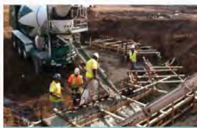
Secured $16M to implement the HUB park and flood control project. Completed 90% of construction activities as of November 2015.
