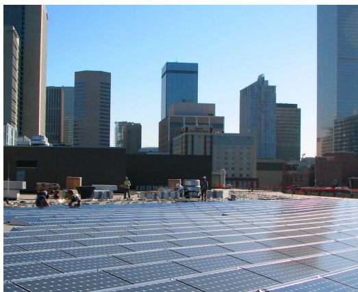
Rooftop solar in Denver, CO. Credit: National Renewable Energy Laboratory
