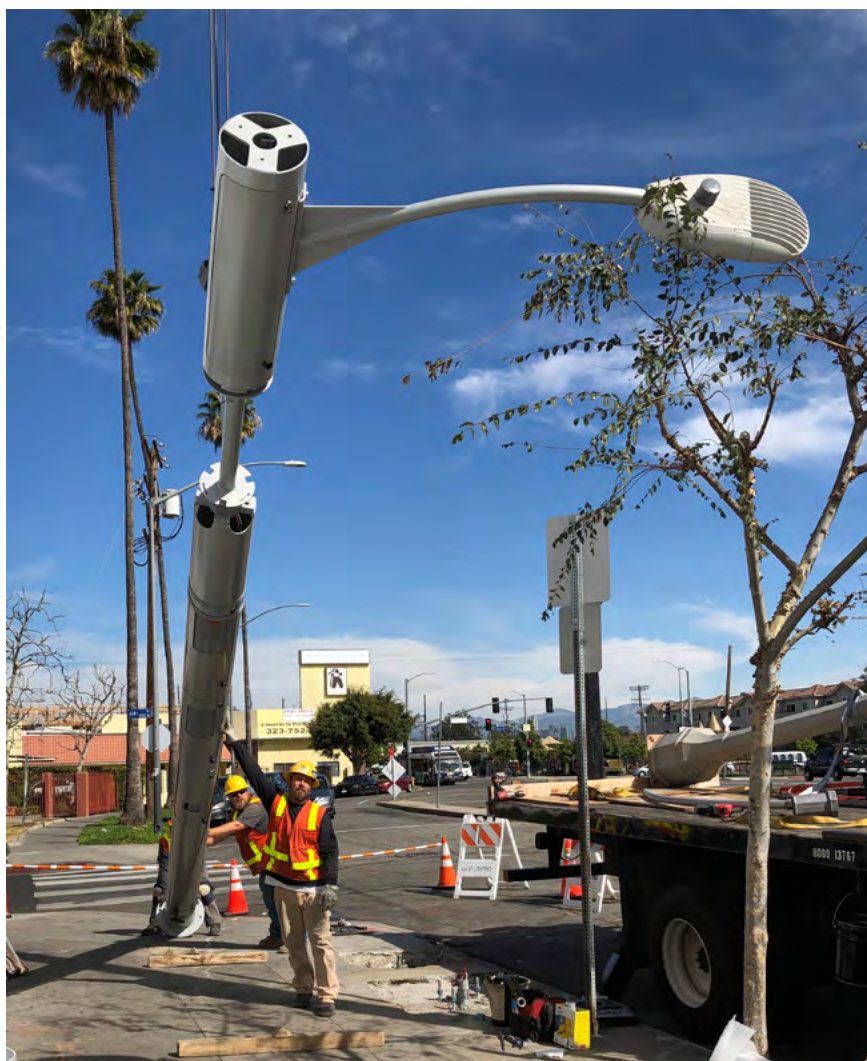
Figure 5.3. Los Angeles’ smart streetlights (Los Angeles Bureau of Street Lighting)
