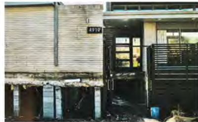
Construction photo showing house elevating on extended foundations. Spaces below SLR-DFE are not habitable. Office / "Mid-Century Elevated: How an Architecturally Significant House Was Lifted Above the Floodplain" / All photos by Raj Mankad
